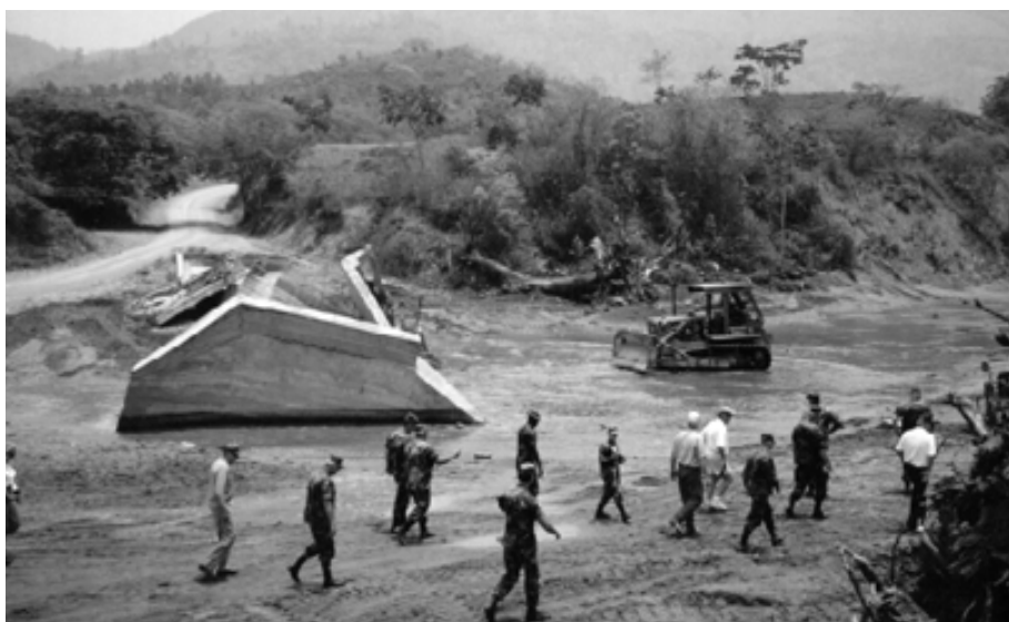
An ARNG bulldozer installs culverts over Rio San Juan in Honduras during Exercise New Horizons.
