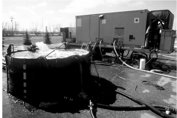
Reverse Osmosis Water Purification Units provide a reliable way to purify water.
